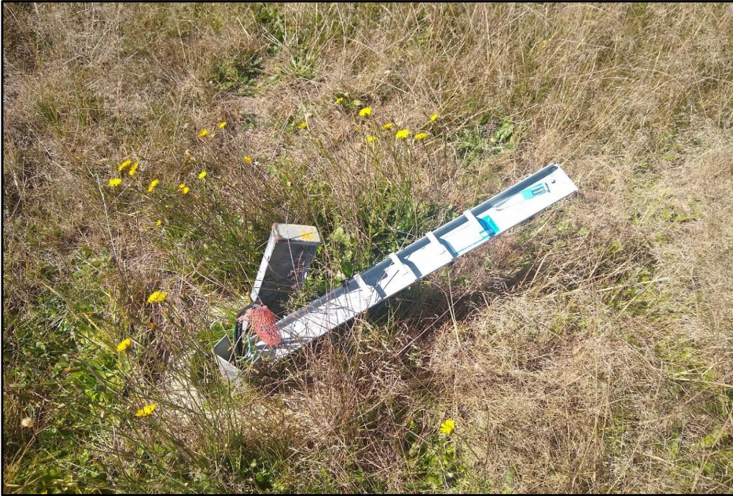
Photo 15: View of disconnected Telstra service
